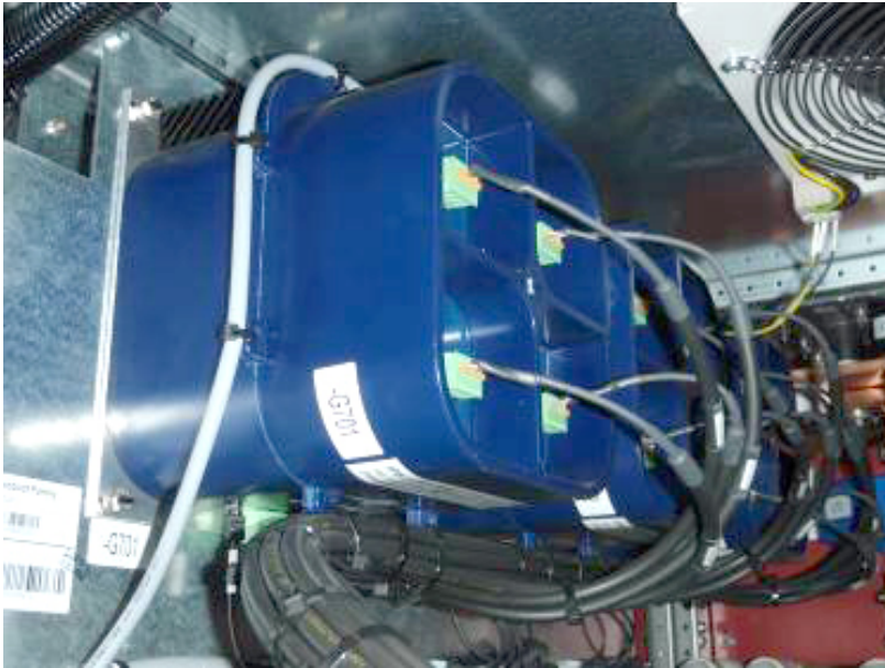
Figure 9–17 IGCT power supply (IPS)
