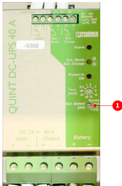
Figure 8-2 UPS -G302 selector switch “Bat.-Select”
