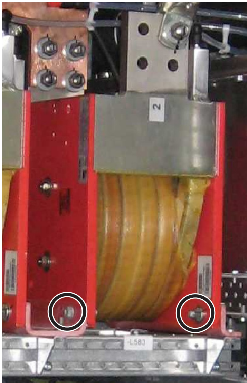
Figure 10–54 dv/dt filter reactor mounting bolts (different VFM variants)
