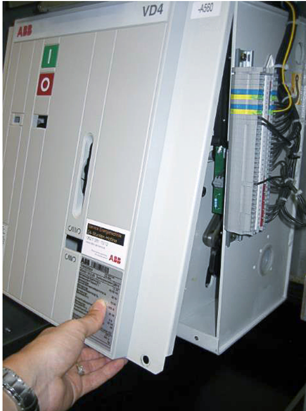
Figure 10–117 Breaker's protecting earth connection
