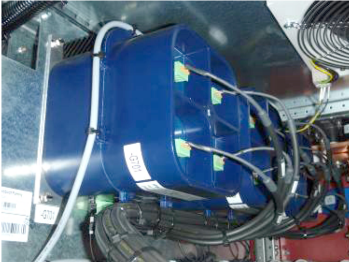
Figure 8–12 GCT power supply (IPS)
