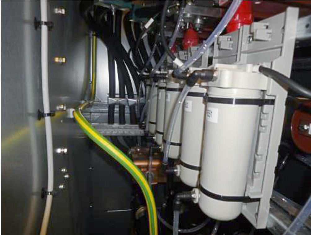
Figure 10-131 dv/dt filter resistors
