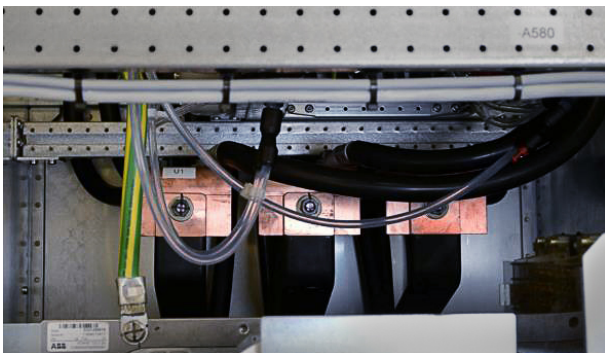
Figure 10-114 Breaker's upper power cable connection
