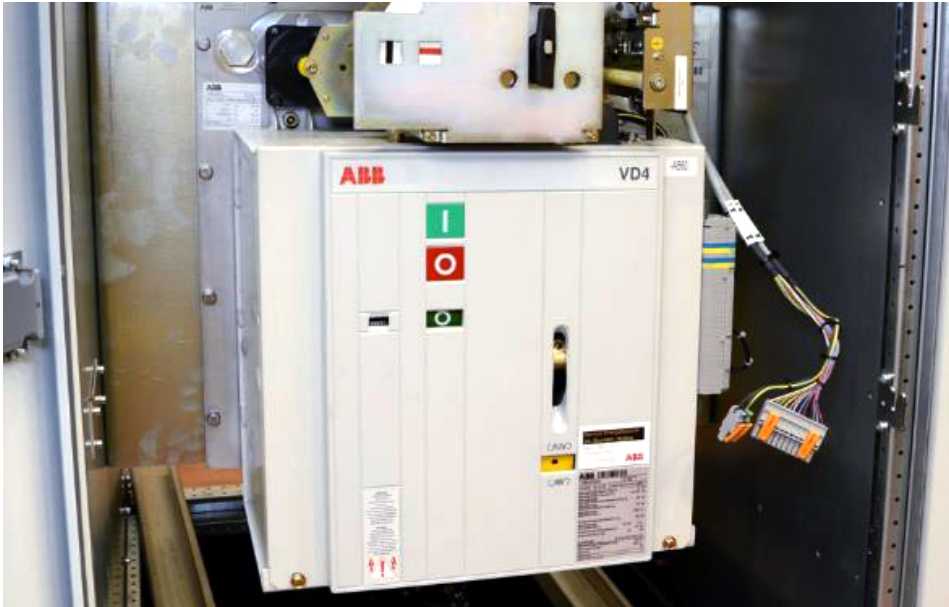
Figure 10-104 Generator breaker (GEB)
