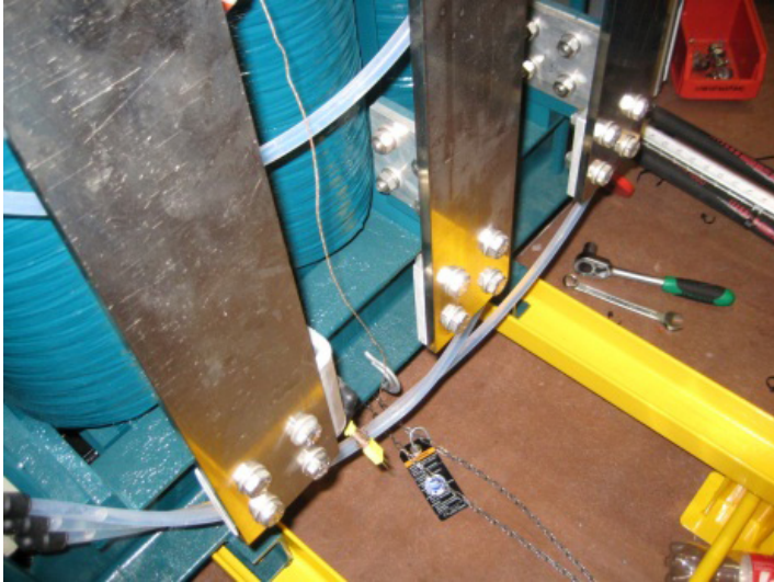
Figure 10-100 Removed filter reactor
