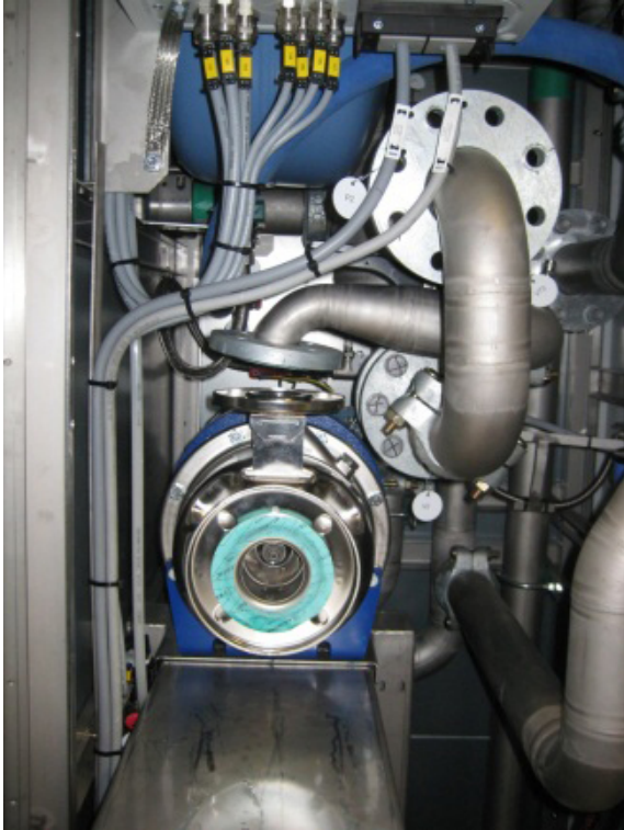
Figure 10–77 Connecting pipes turned aside
