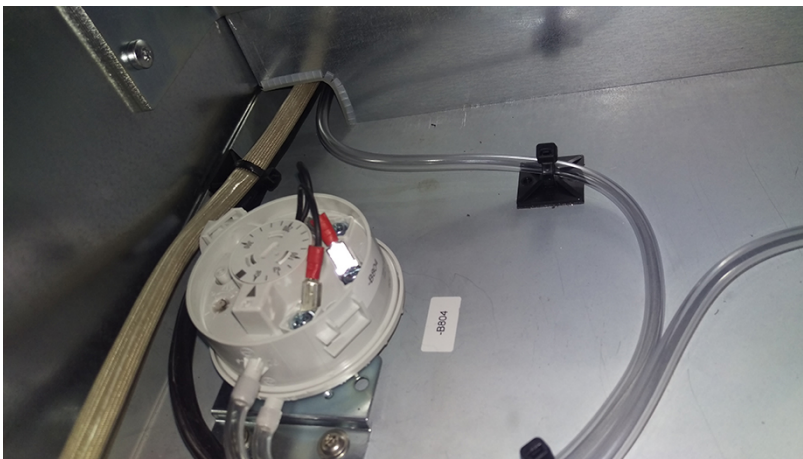
Figure 10–110 Differential pressure measurement device
