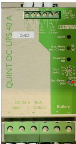
Figure 8-11 UPS -G402 selector switch “Bat.-Select”
