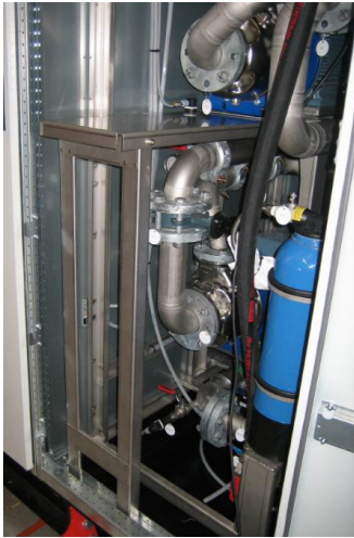
Figure 10–79 Pump maintenance table with long legs (for upper pump)
