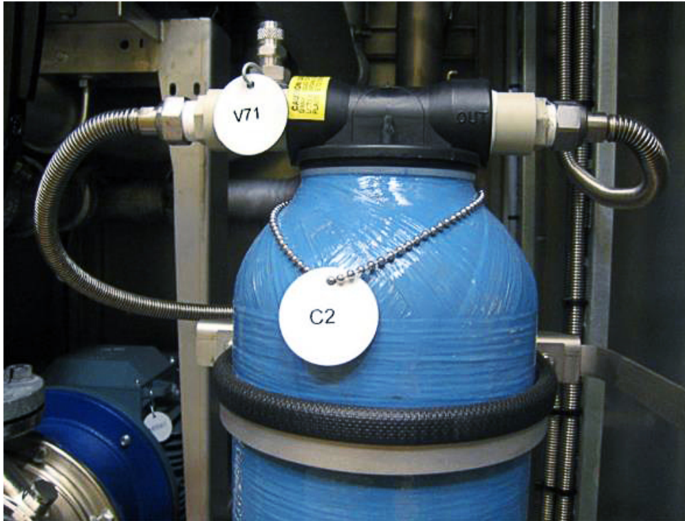
Figure 10-73 Ion exchange vessel
